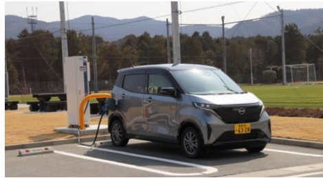
EV charging station
